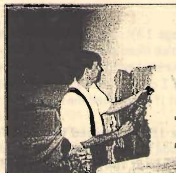
Mr. Christian Nelson cuts a hole in the wall to create a new entrance for the office.
